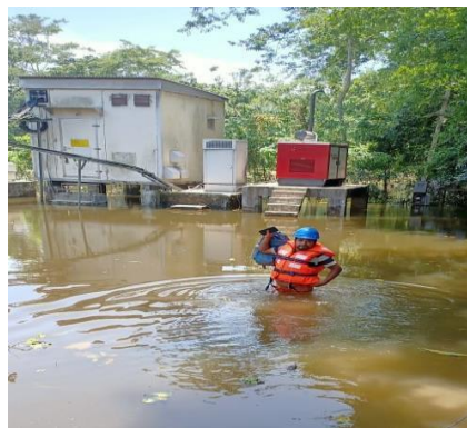
Network restoration efforts during floods in Assam
